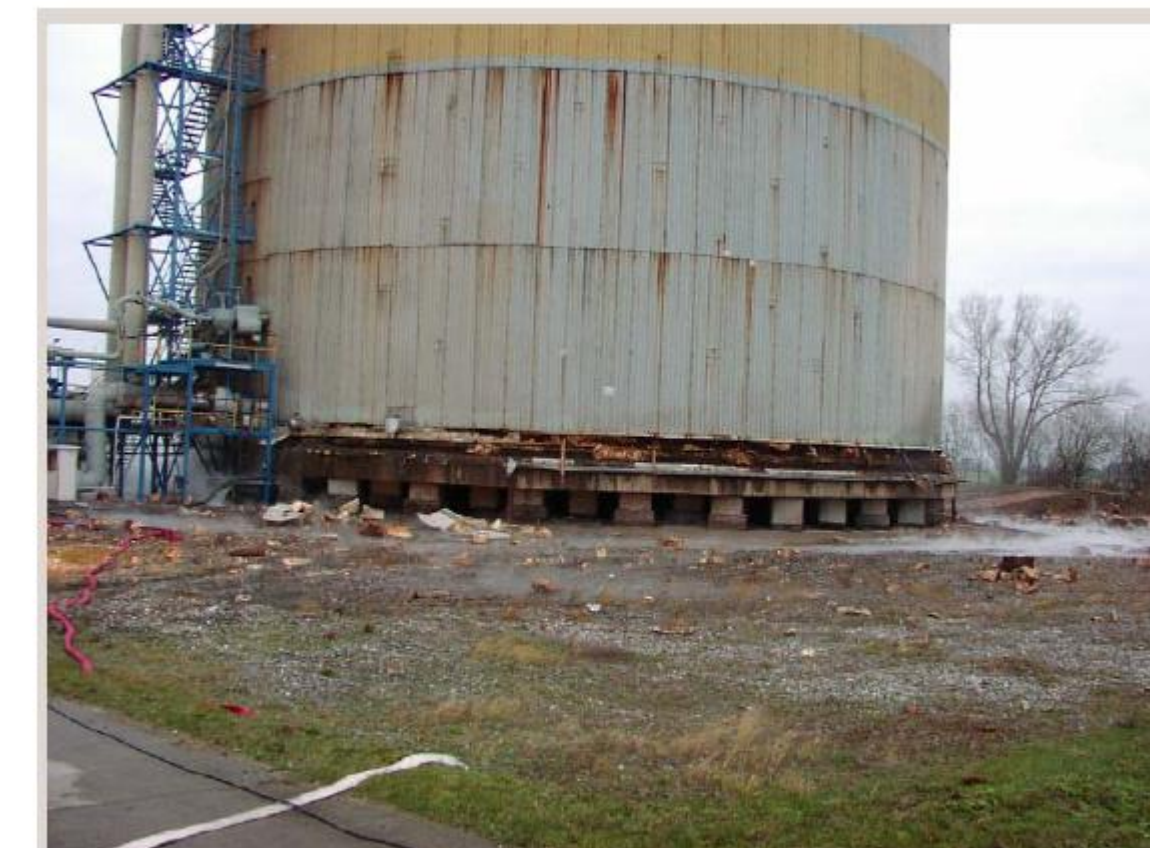
Figure 4 Yara Rostock tank after the accident.
